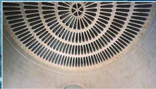
Self-supporting stepped dome grid in an absorption tower.
