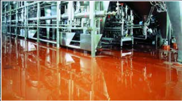
Floor coating in a chemical plant.
