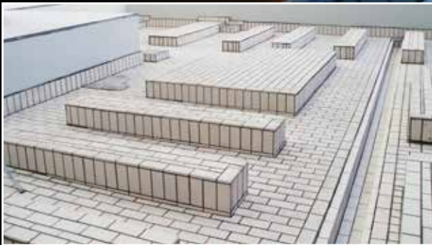
Combined lining system composed of sealing membrane and ceramic tiles in a containment basin.
