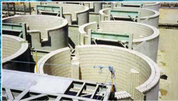
System lining with ceramic bricks.
